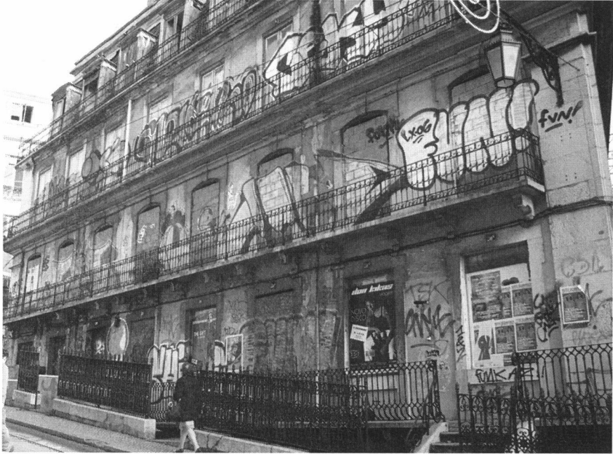
FIGURE 2 Street Bombing on Abandoned Buildings (Lisbon, 2009)
